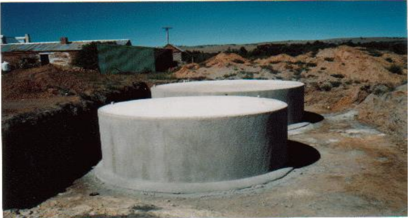
Figure A: Large Scale Capture and Use Tank
