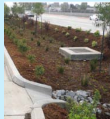
An overflow outlet conveys runoff that exceeds the bioretention area capacity.
