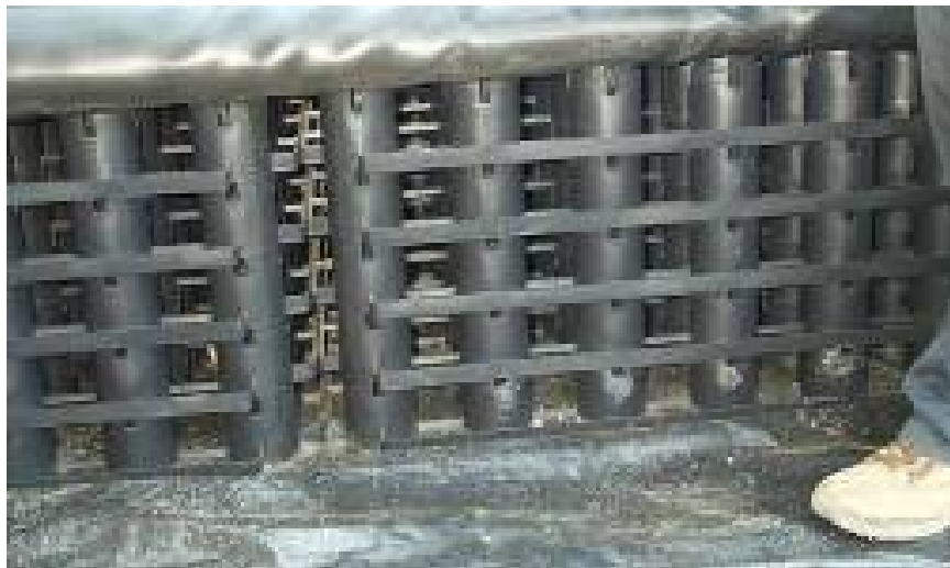
Figure 67. Rainstore™ units used as the storage element underneath a brick pathway atop a vegetated rooftop plaza. Source: Cahill Associates
