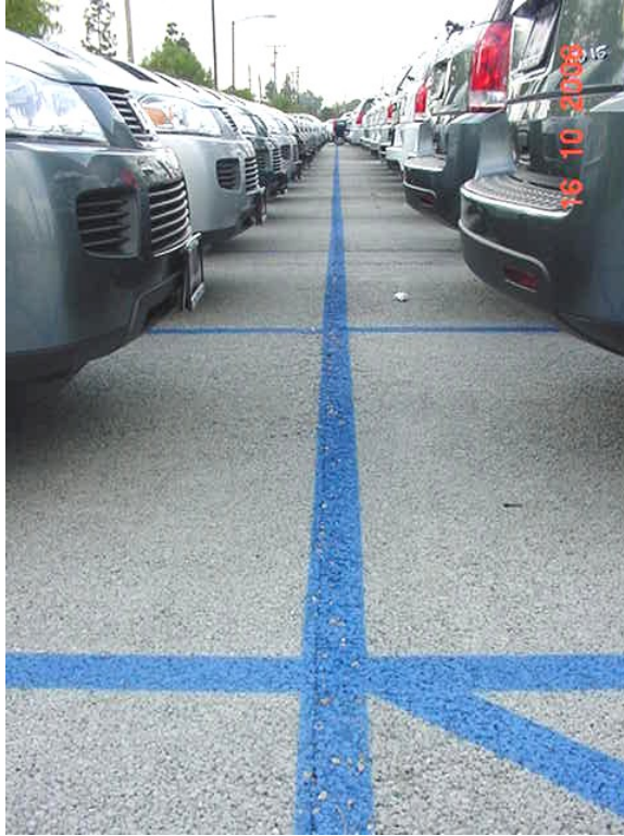
Figure 42. Pervious concrete in Cerritos, CA. Source: Bill DePoto
