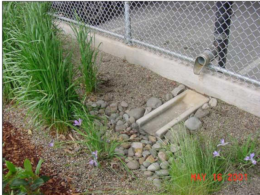
Figure 72. Downspout disconnection into vegetated area. Source: Prince George's County, MD Department of Environmental Resources
