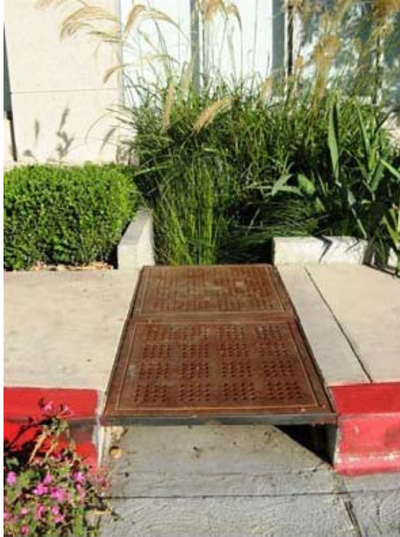
Figure 25. Curb cut directing water from the street into a bioswale. Source: Haan-Fawn Chau
