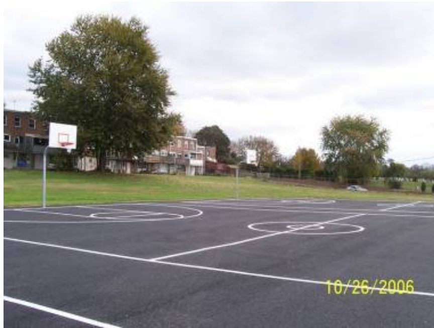
Figure 36. Pervious asphalt basketball court at 2nd Ward Neighborhood Park in Upper Darby, PA. Source: Cahill Associates
