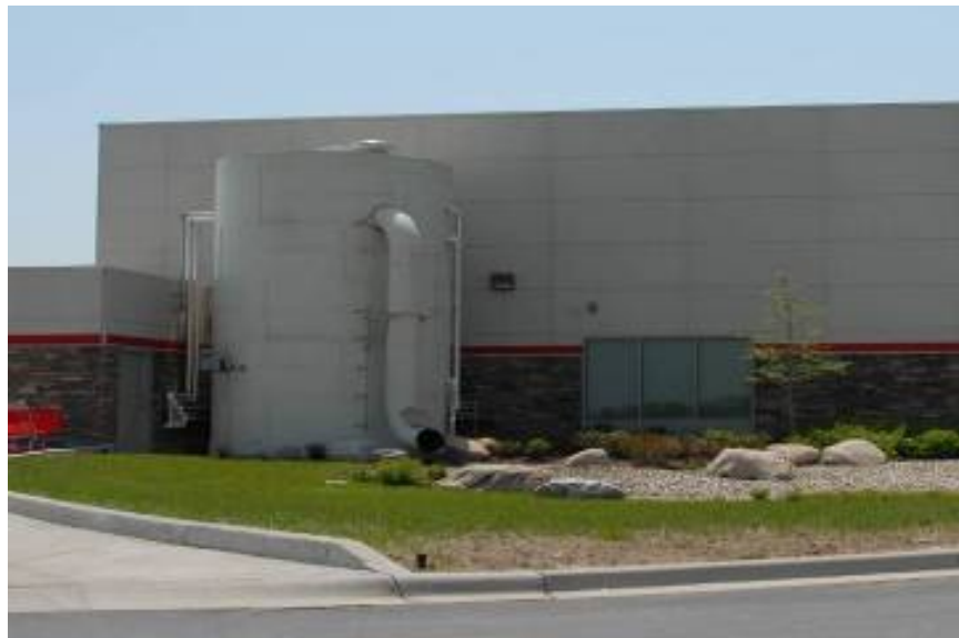
Figure 60. Outdoor Cistern with Overflow Directed to Pervious Area. Source: SEMCOG
