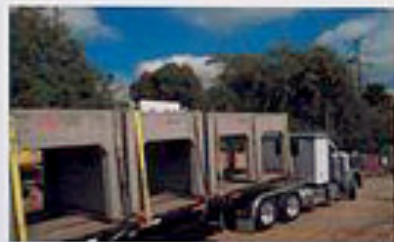
Two large culverts have been installed to capture runoff from the park's storm drain. The culverts are made up of modular units shown here during installation.
