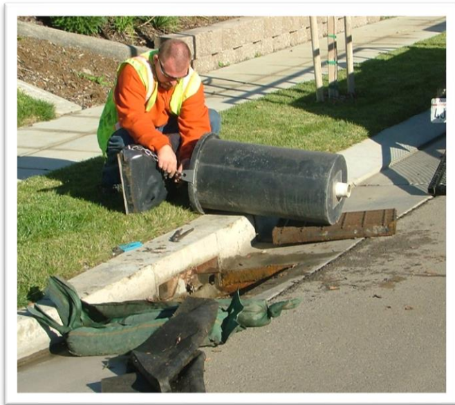
Image 7: Installation of an original unit on a side inlet. (Unit can be easily modified to meet trash capture requirements)
