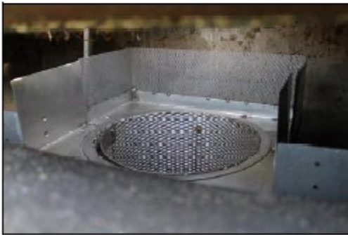
Figure 21 - Curb Inlet Filter Basket Installed In Tray System.
