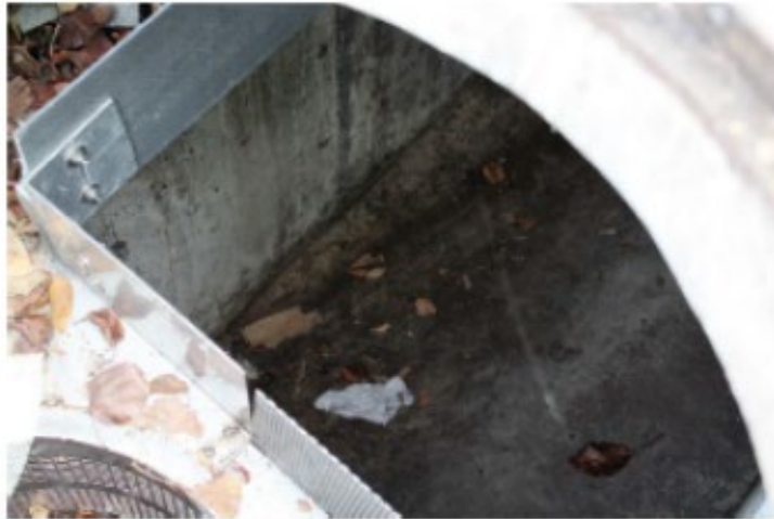
Figure 26 - View 3 of Catch Basin Bottom with Bio Clean® Curb Inlet Filter Installed
