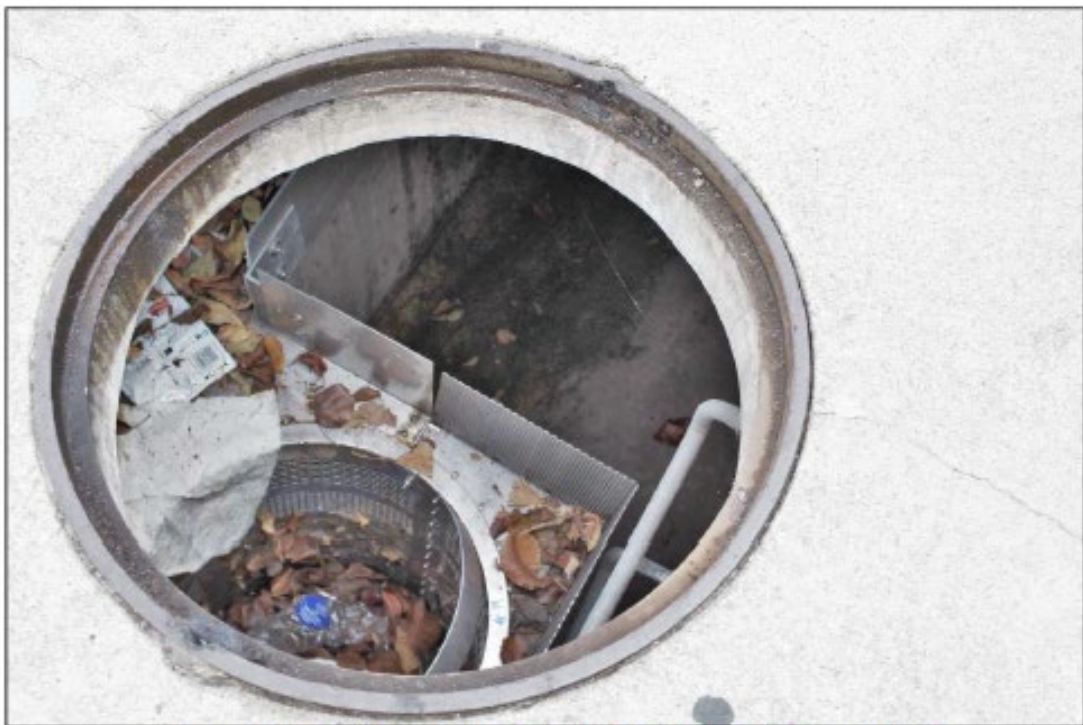
Figure 25 - View 2 of Catch Basin Bottom with Bio Clean® Curb Inlet Filter Installed
