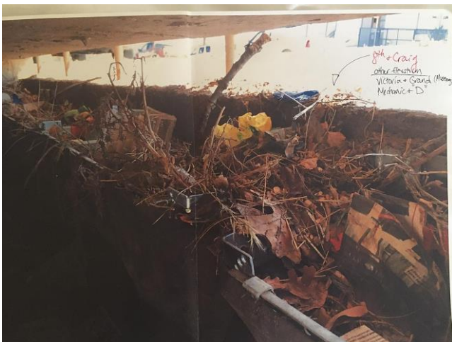
Photo 4: Improperly maintained Open Throat Curb Inlet Filter in Pueblo, Colorado.
