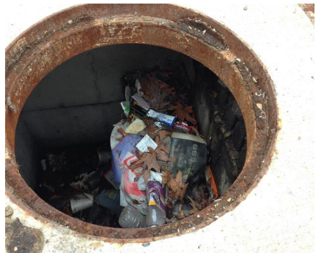
Photo 5: Philadelphia Water Dept. Wall Mount Filter where service was overdue
