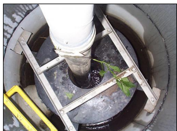
Figure 8 - Defender® During Maintenance
