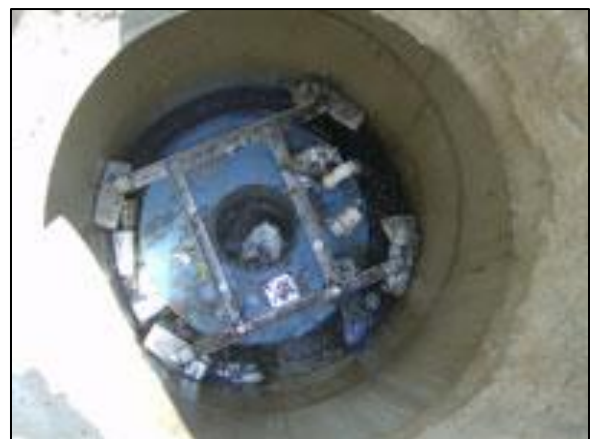
Figure 7 - Defender® In Operation
