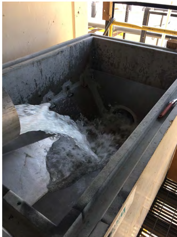
Figure 6. Water flowing into the U/S Sampling Chamber.
