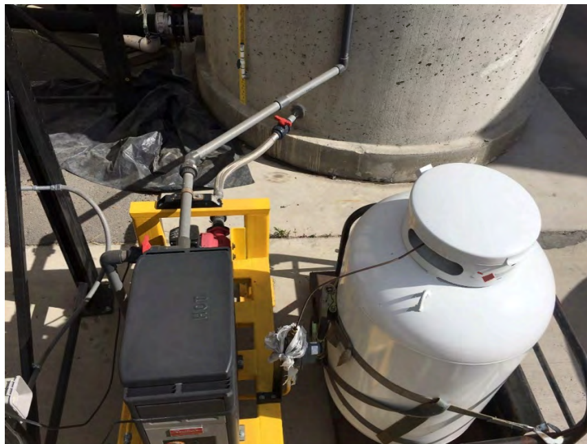
Figure 8. Water heating system and propane tank.
