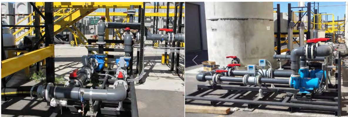
Figure 2. Supply Pump Skid (left) and Return Pump Skid (right).
