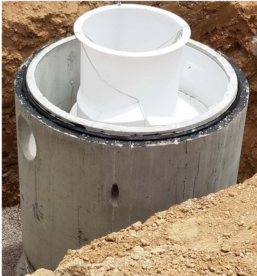
Figure 13. JDS60-2424 Unit Set in Field, Waiting for Riser Barrels and Top Slab to be Stacked to Finished Grade.
