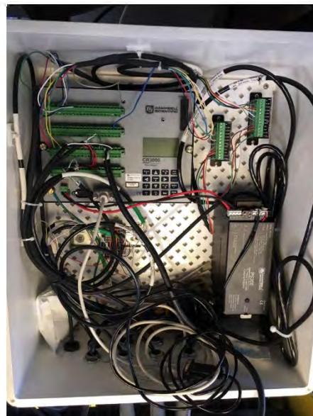
Figure 5. CR3000 DataLogger housed within a weatherproof box.
