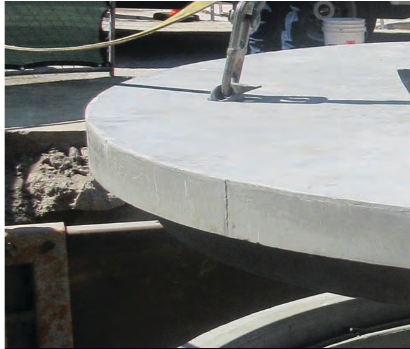
The JDS deployed in underground manholes or
