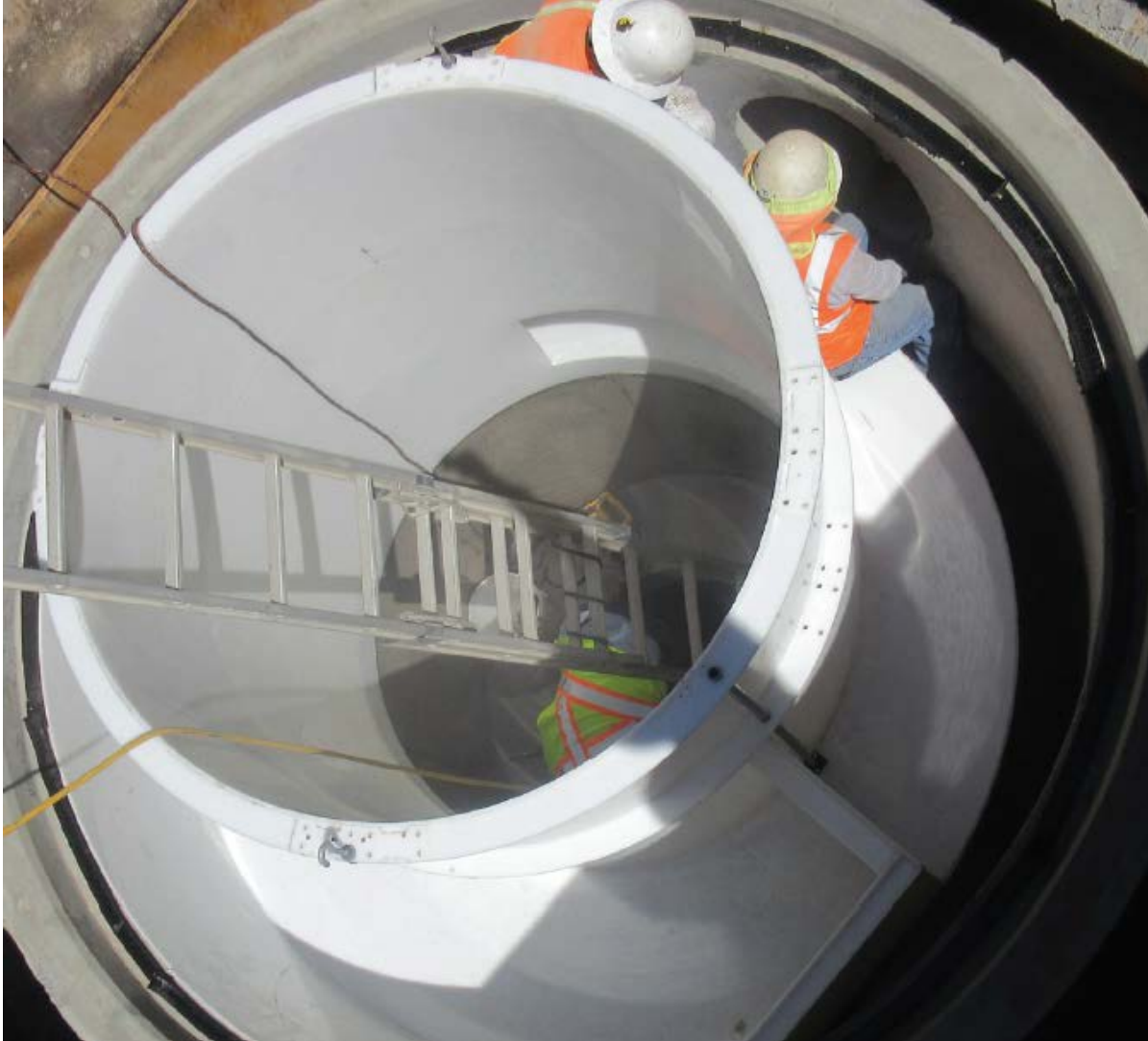
Figure 14. 3x Man Jensen Field Crew Installing the SS Screen Cylinder & HDPE Inlet on a 9-cfs Capacity Inline JDS120-6448 after 120-in ID Manhole Deployment Structure was Set by the Contractor.
