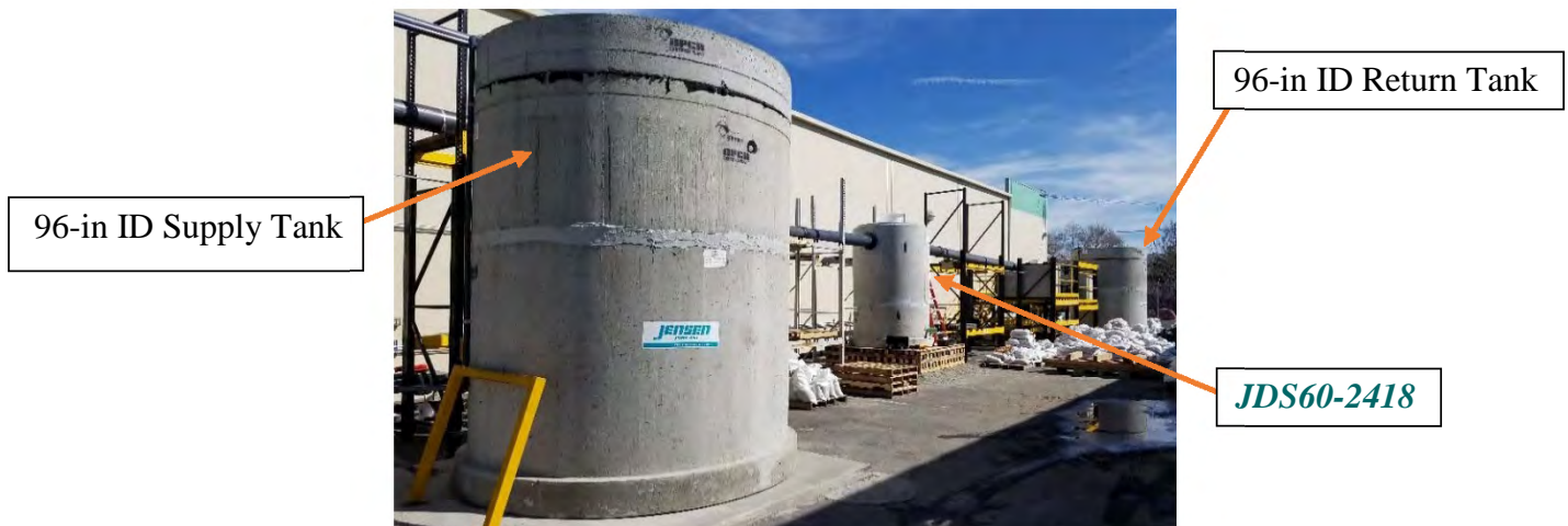
Figure 1. Supply Tank in the foreground with the JDS60-2418 and Return Tank in the background.
