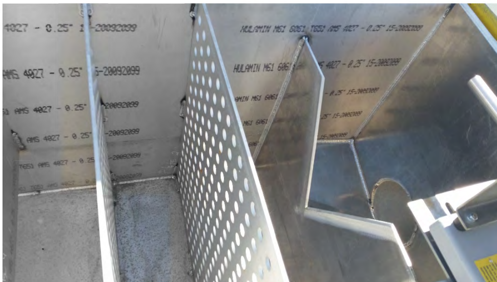
Figure 4. V-notch weir used for flow measurement.
