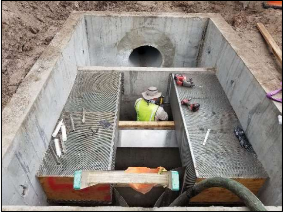
Figure 12 - View of DSBB Screen Storage Chambers
