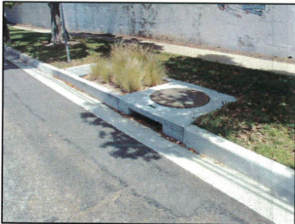
Figure 12 - Modular Wetlands® in Operation
