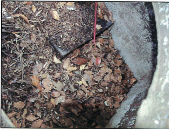
Figure 14 - Pre-Treatment Chamber with Trash and Debris
