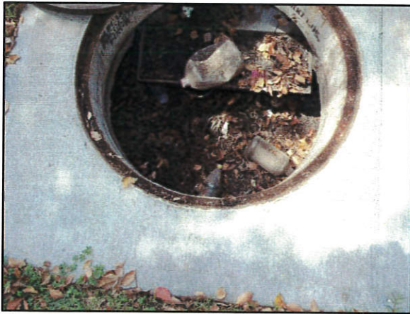
Figure 13 - View of Pre-Treatment Chamber
