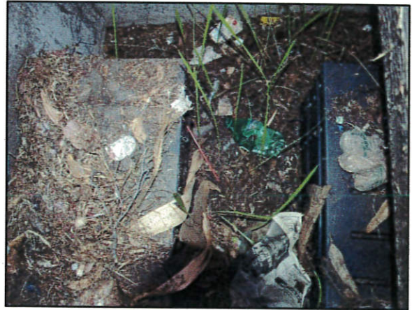
Figure 15 - Pre-Treatment Chamber with Trash and Debris
