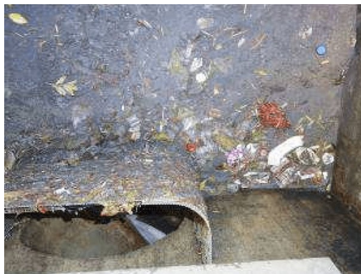
Figure 6 – CPS Prior to Maintenance (U-Shaped)
