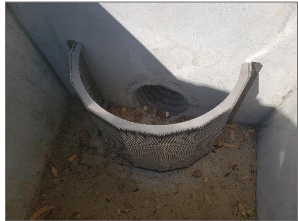
Figure 10 - CPS Installed - Top View
