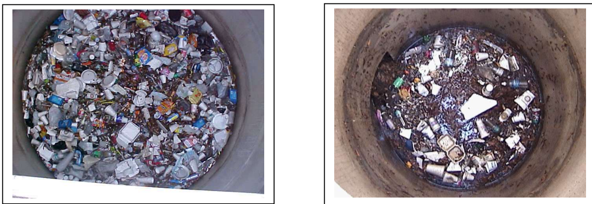
Figure 8 - Gross Pollutants Captured in the CDS Units Sump
