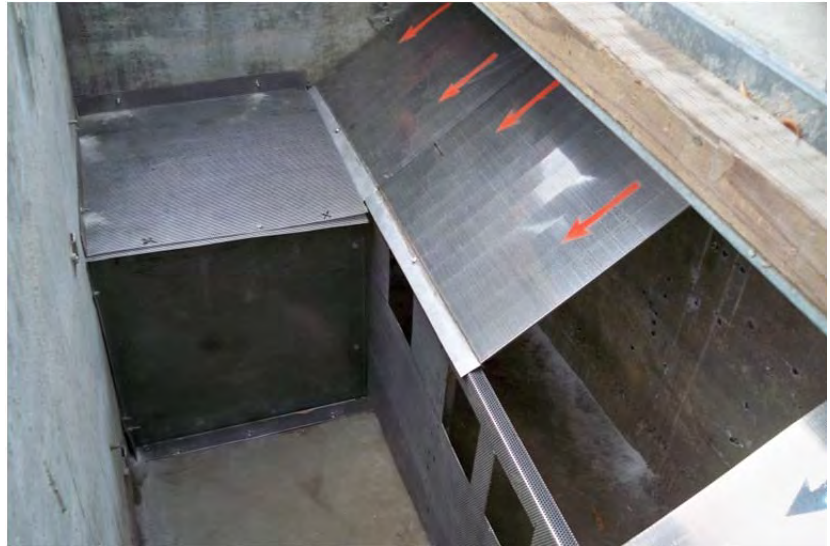
Figure 1 - Coanda Installation at LA County Test Facility
