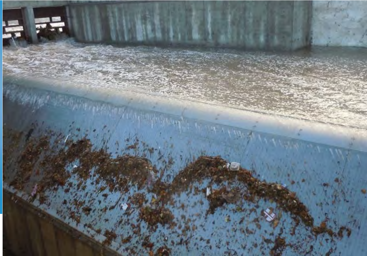
Coanda-effect screen application at Storm water Quality Facility, Albuquerque, New Mexico. Ho and Daggett (2011) AWRA conference.
