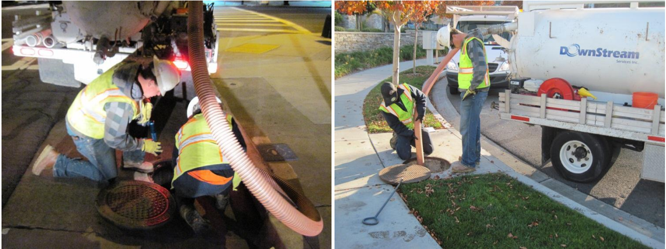
Figure 7. Vactor clean-out by Downstream Services, Inc. in the Downtown and Scripps-Poway areas.
