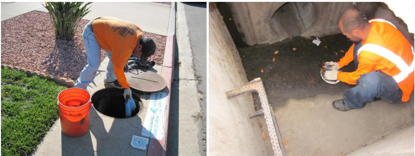
Figure 6. Manual clean-out by Ron's Maintenance in the Tecolote and San Ysidro areas.
