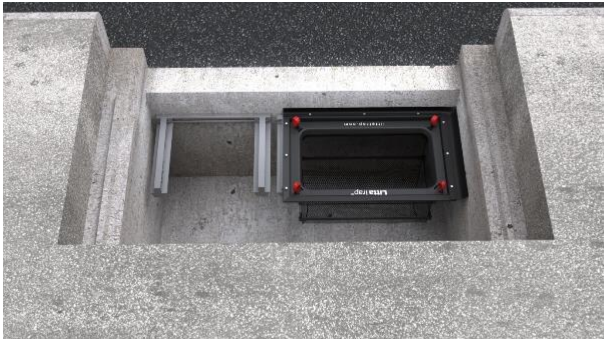
Figure 7: Installation of LTFC9060 LittaTrap FC and bracket for LTFC6060 in Curb Entry Catch basin
