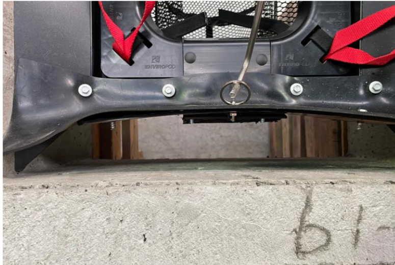
Figure 16: Enviropod® LittaTrap™ with Vector Inspection in open position.
