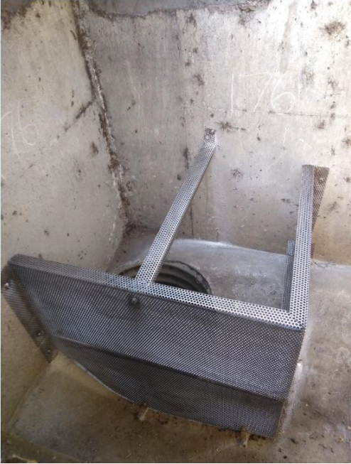
Floor discharge pipe - G2-1 CPS-Mod™
