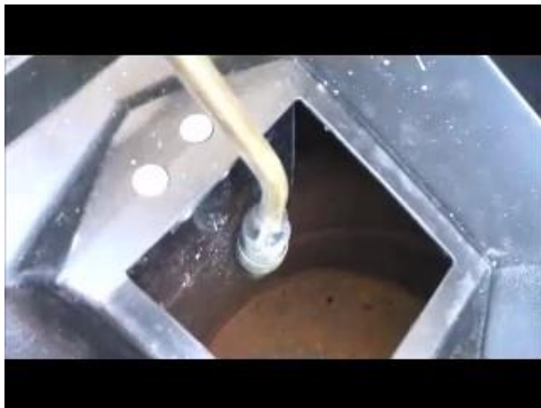
From left to right, top to bottom: Nozzle hose accessing viewport through grate, technician lifting grate to illustrate nozzle inside viewport for inspection.
