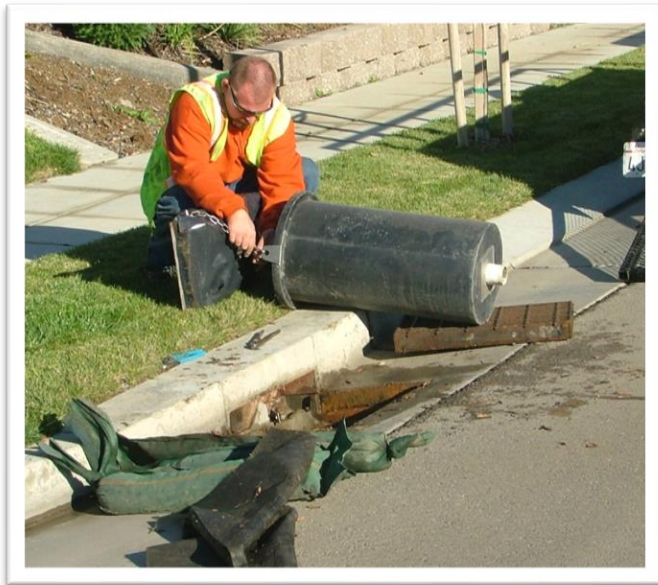
Image 1: Installation of an original unit on a side inlet. (Unit can be easily modified to meet trash capture requirements)
