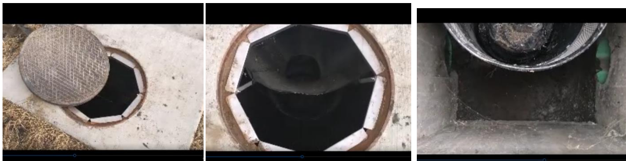
From left to right: Curbside inlet has ample room to view bottom of catch basin, no obstructions.
