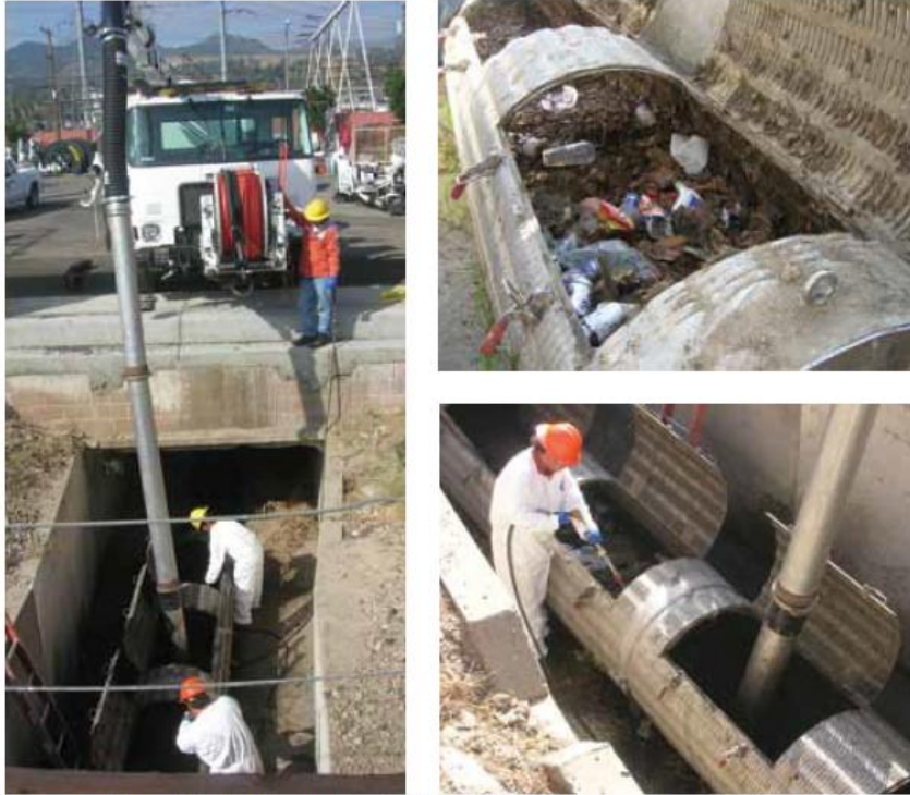
Screens are quickly and effectively cleaned with combined use of a high pressure hose and vacuum equipment.
