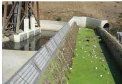
Pump station with array of louver panel screens.
