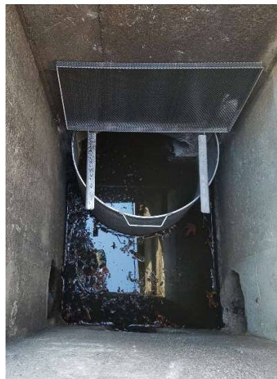
Figure 6. Lid lifted for access.
