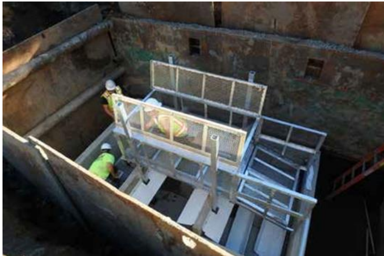
Base section set in excavation with sediment chamber baffle walls, turbulence deflectors, and screen basket system installed. Screen basket system cover shown in open position.
