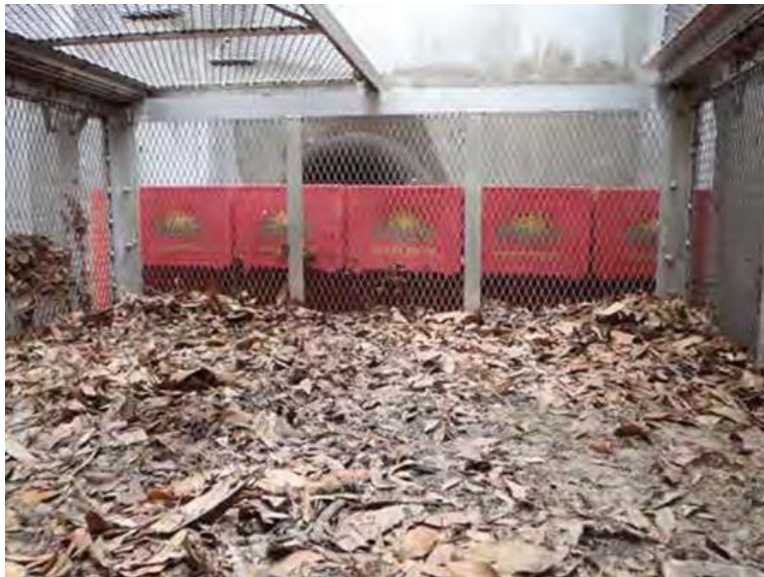
Active installation. Trash and debris shown captured in the screen basket system. Left side of screen basket system cover shown in closed position and right side of screen basket system shown in open position. Both sides can be opened to facilitate maintenance.
