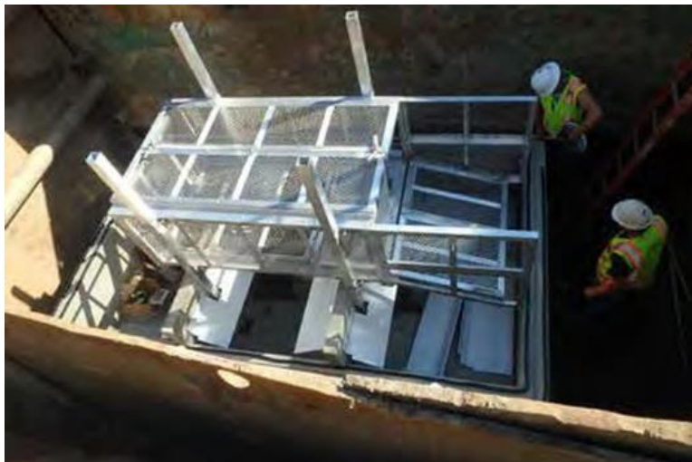
Base section set in excavation with sediment chamber baffle walls, turbulence deflectors, and screen basket system installed. Screen basket system cover shown in closed position.
