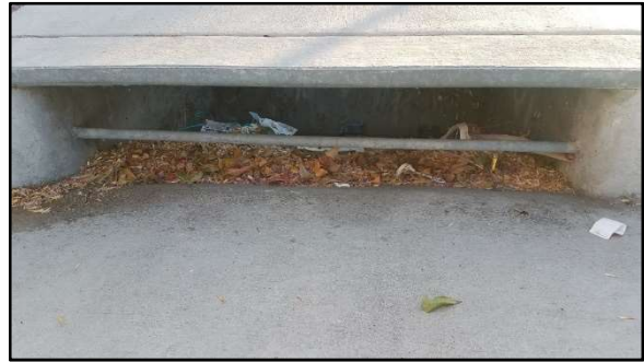
Figure 2. Installed FloGard® CIB – full (view from curb).
