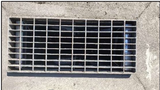
Figure 3. Installed FloGard® GIB with grate.
