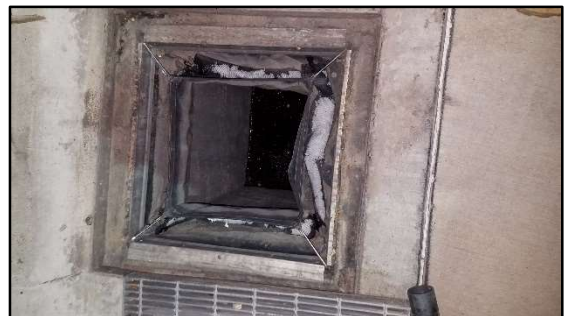
Figure 6. Installed FloGard® GIB – view to bottom: water.
