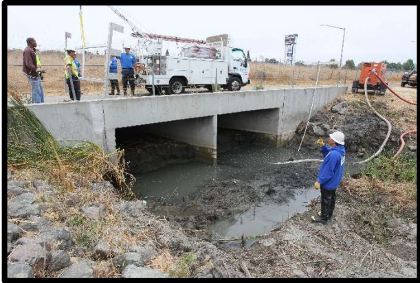
Figure 8. Regional trash capture project.
