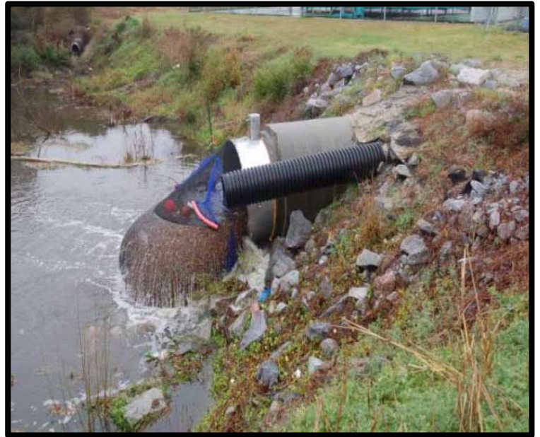
Figure 2. Routine inspection 2 months post-installation. Maintenance to be performed.
