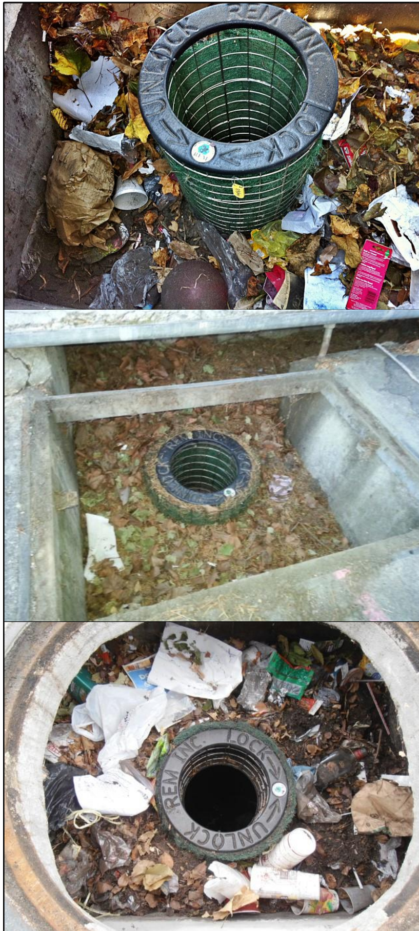
Photos of three test units previously installed.
