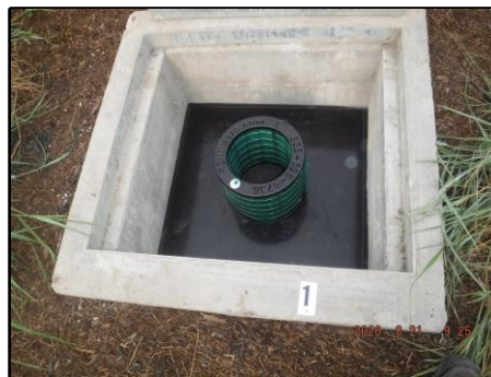
Model: TR3636-TH Installed
