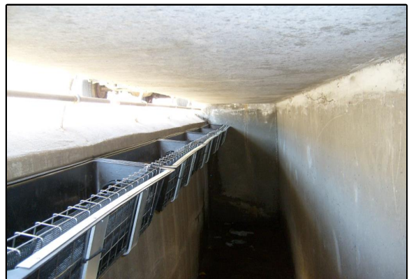
Model: TRC21.0 Installed
