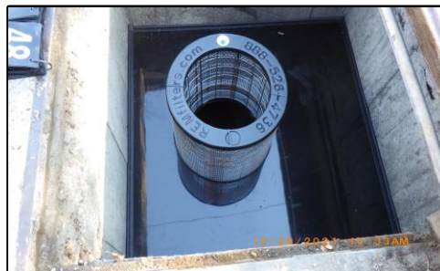
Model: TR3636-TH-PERF Installed
