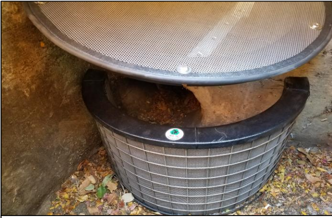
Test Unit T3: TR24(16)-CPS 1 Week after installation
