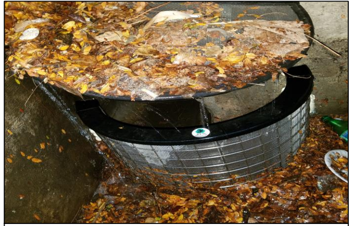
Test Unit T3: TR24(16)-CPS Rain Event 2 months after installation – 25% Capacity
