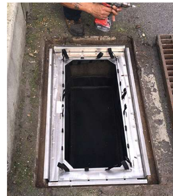
Installed Fabco StormSack
