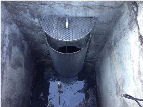
Figure 1. Installed Stormtek device
