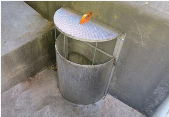
Figure 2. Installed Stormtek device
