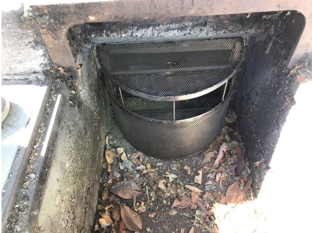
Figure 6. Installed Stormtek device in shallow sump
