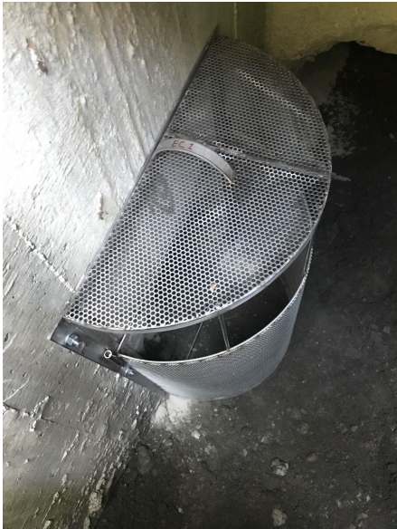
Figure 3. Installed Stormtek device
