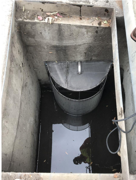
Figure 4. Installed Stormtek device
