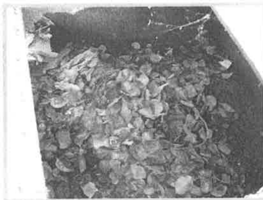
Figure 3.2 Typical CB insert with vegetation in catchment area
