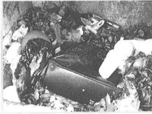
Figure 3.1 Typical CB insert with trash in catchment area
