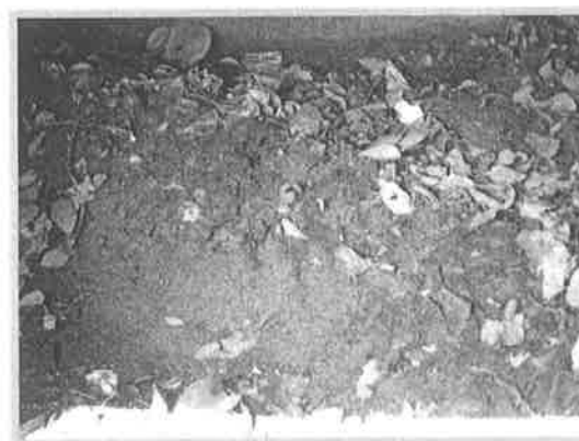
Figure 3.3 Typical CB insert with sediment in catchment area
