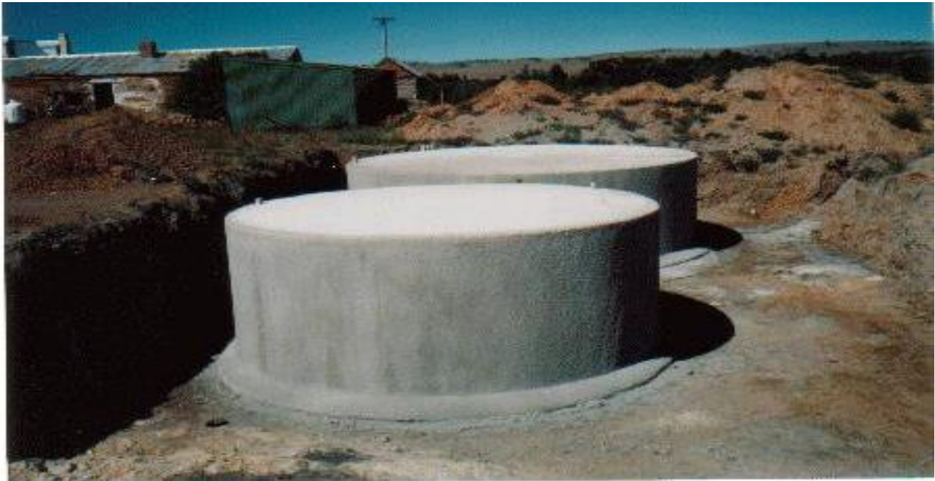
Photograph of a Large Scale Capture and Use Tank
